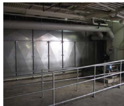
300kL rainwater harvesting tank
