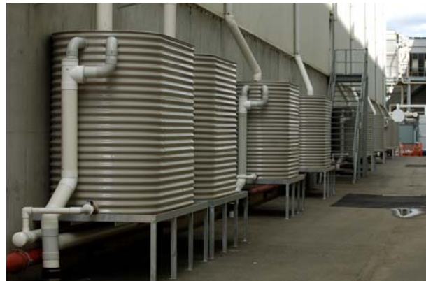
One component of Cadbury's series of rainwater tanks
