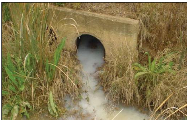
Domestic greywater entering a waterway from the drainage system
